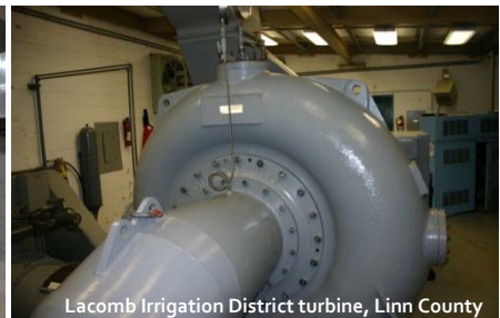
Lacombe Irrigation District turbine, Linn County
