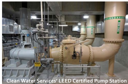
Clean Water Services' LEED Certified Pump Station
