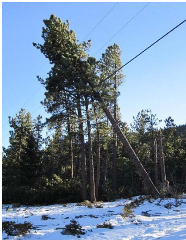
Tree felled by wind leans against a transmission line in the San Isabel National Forest in Colorado.
